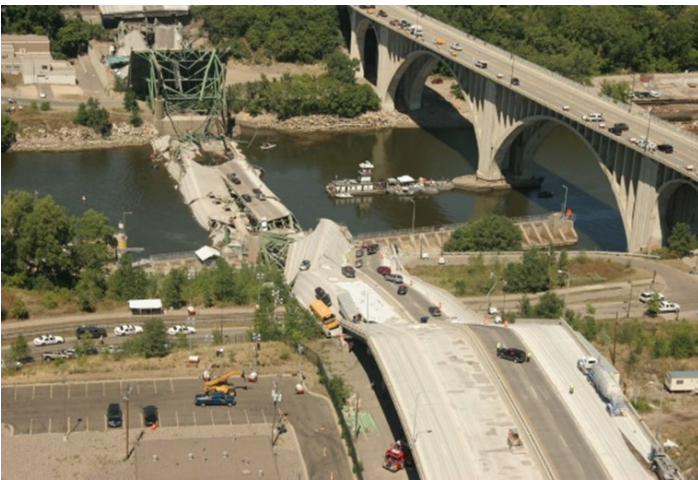
Figure 1: The I-35W Mississippi River Bridge, which catastrophically failed during the evening rush hour on August 1, 2007
